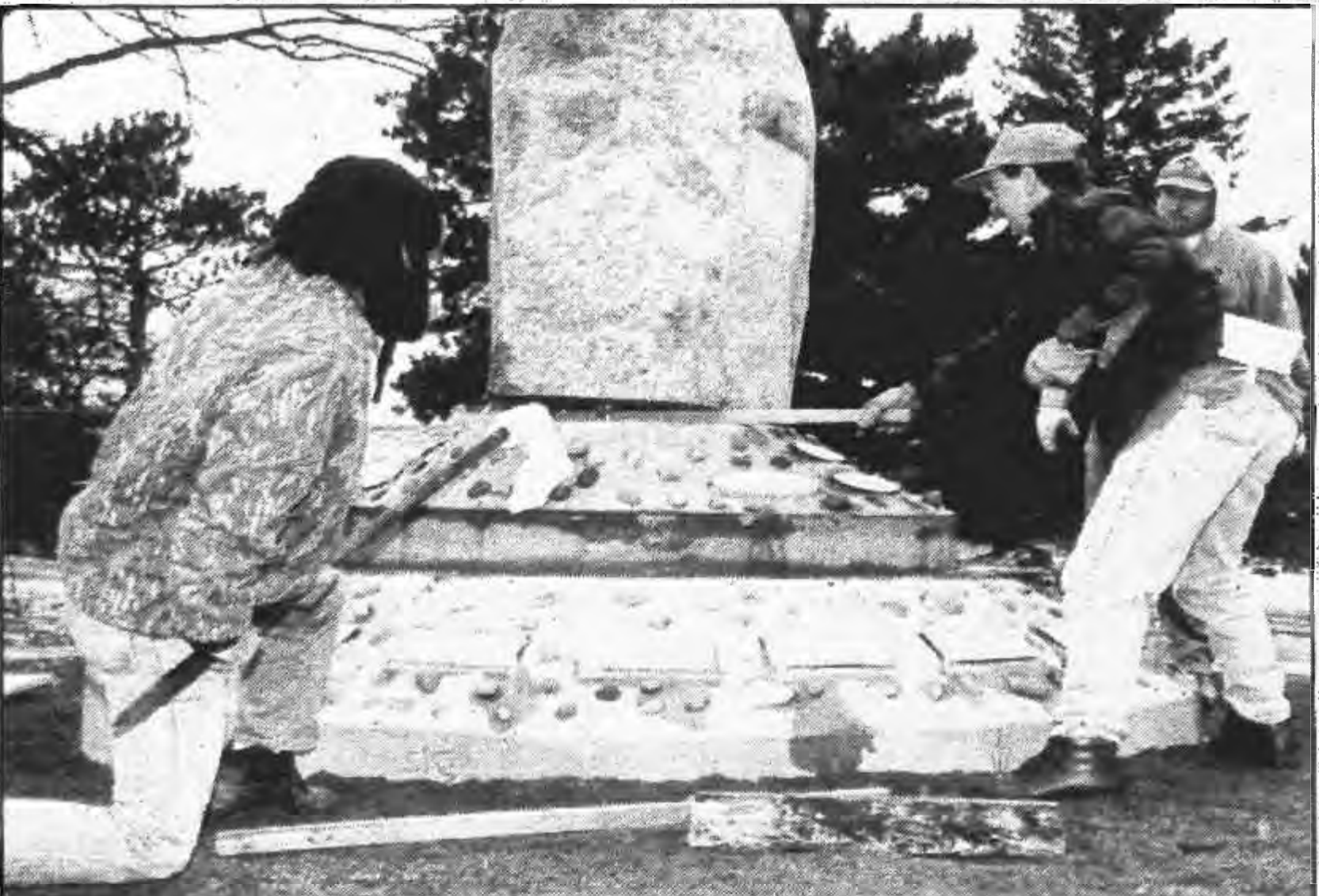
The Mikwendaagoziwag Memorial Monument begins to take shape with Grandfather stones brought from 11 Ojibwe reservations embedded in the base. Above, Bruce Goman, Mille Lacs Development, Inc. and Jim Zorn, GLIFWC policy analyst, work with the St. Croix construction crew to place the giant boulder on the monument's base. (Photo by Charlie Otto Rasmussen)
