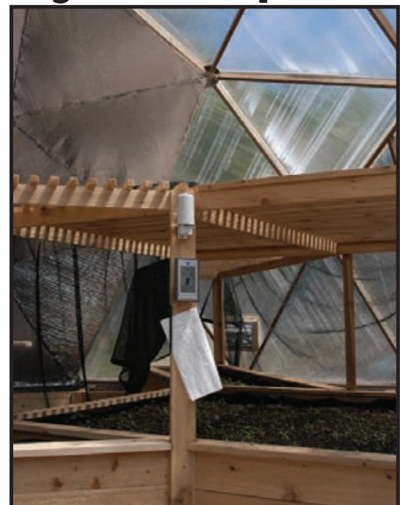
KBIC's new native plant greenhouse was constructed with help from volunteers and a number of groups, including teens enrolled in the KBIC youth program. (COR)
