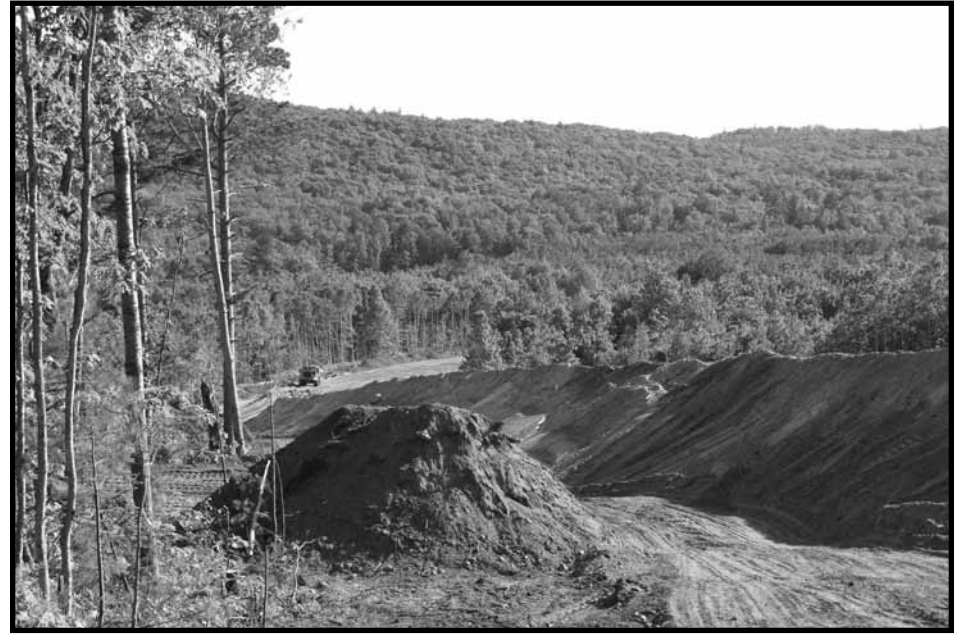
Photo 2—Eagle mine haul road has caused habitat fragmentation in this biologically rich area.
