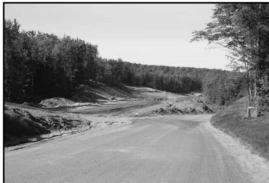
Photo 1—Eagle mine haul road under construction. No evidence of silt fencing or erosion control best management practices are visible.
