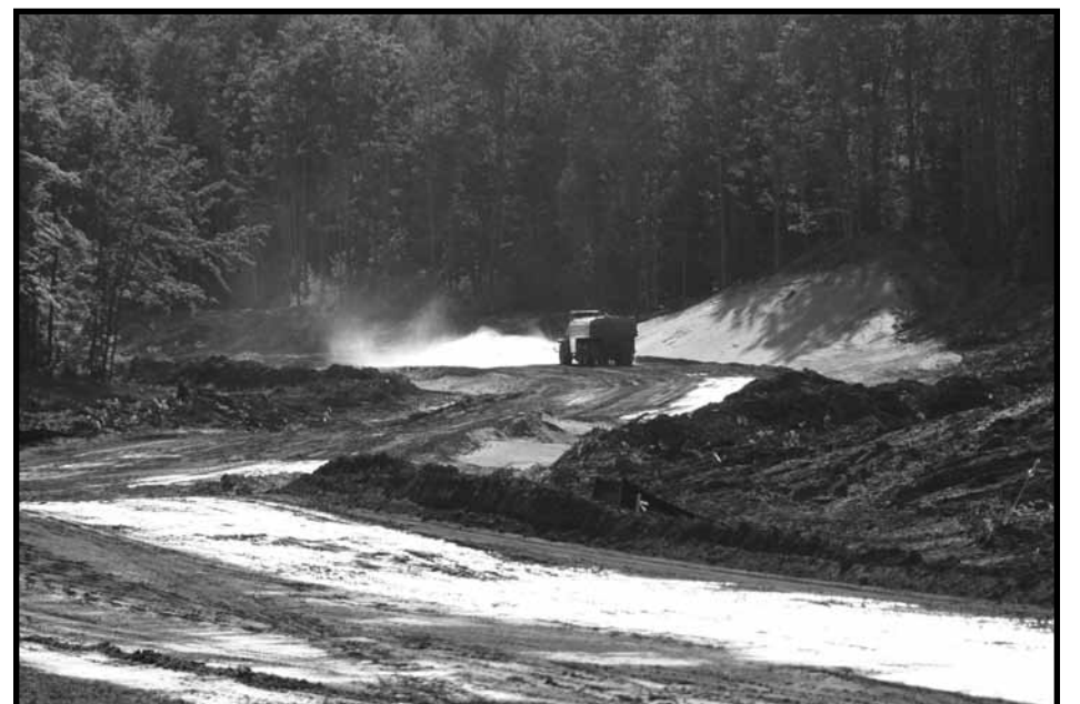
Photo 3—Tanker spraying water for dust control along the Eagle mine haul road construction site.
