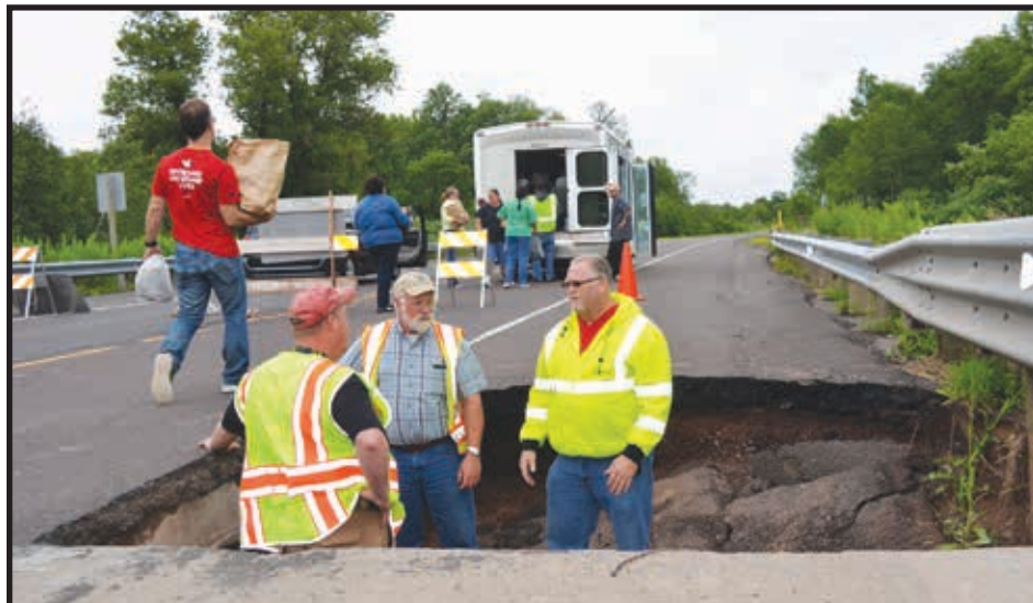
As highway engineers discuss repair plans in a washed out section of US Highway 2, flood relief volunteers hand-carry supplies to waiting vehicles bound for New Odanah July 14. (CO Rasmussen photo)
