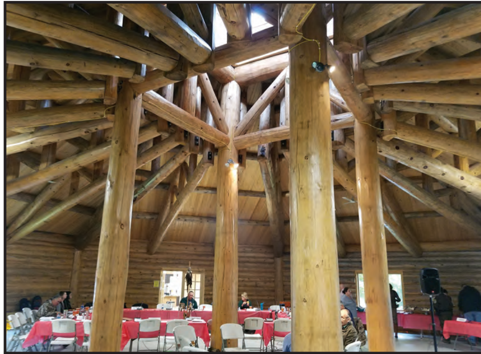
Located at Old Indian Village on the north shore of Vieux Desert Lake, the Lac Vieux Desert traditional roundhouse is built from pine logs acquired through collaborative work with the US Forest Service. The eight-sided structure is made up of approximately 150 twenty-five foot logs, plus eight large, 20-25 inch diameter logs utilized for roof trusses. The federal and native signatories to the Tribal/Forest Service Memorandum of Understanding held their 20th annual meeting at the roundhouse October 3. (P. Strong photo)
