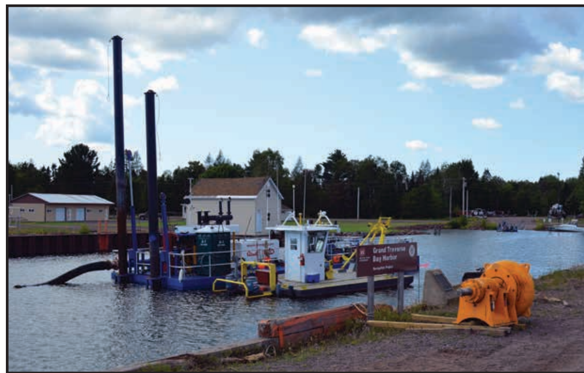
A barge at Grand Traverse Harbor dredged stamp sands from the bottom of the Traverse River last August, sending the mining waste through a 4-mile pipe to an upshore containment area. (CO Rasmussen photo)
