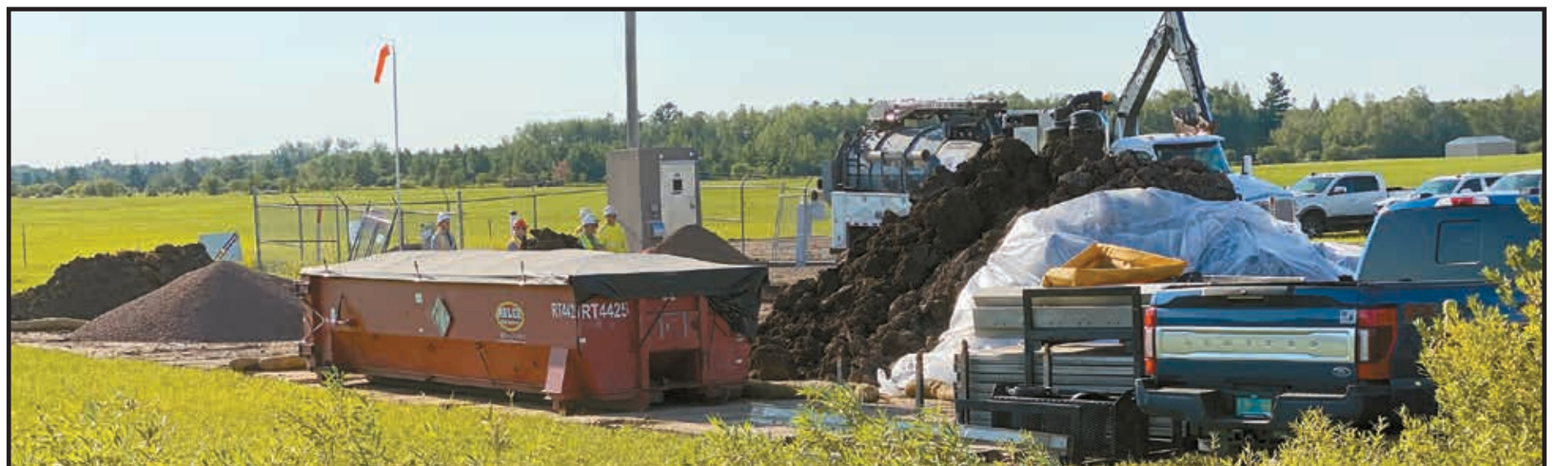
Enbridge crews operate machinery and heavy equipment at the site of a potential Line 5 oil leak just west of the Bad River Reservation August 4. Wisconsin Department of Natural Resources reported that all the suspect soil around the pipeline was excavated and stockpiled. (CO Rasmussen photo)
