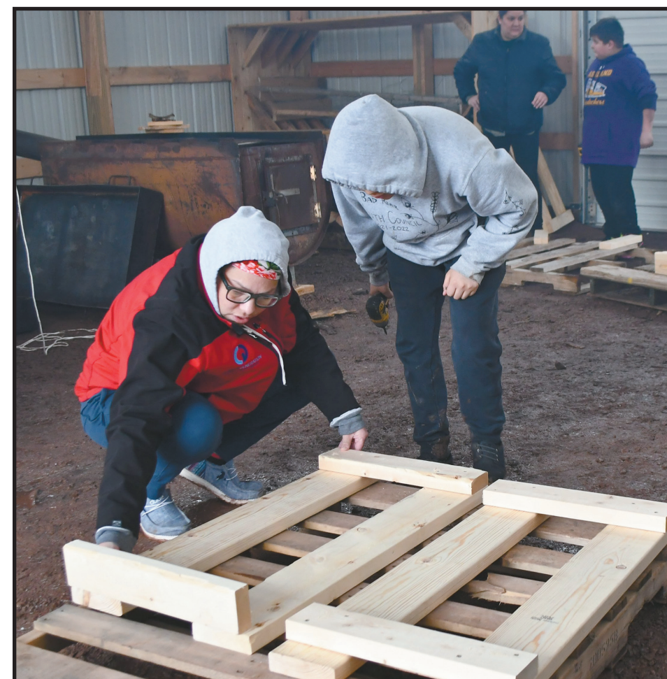
Families worked together to frame-up hand washing stations on April 30. (CO Rasmussen photo)
