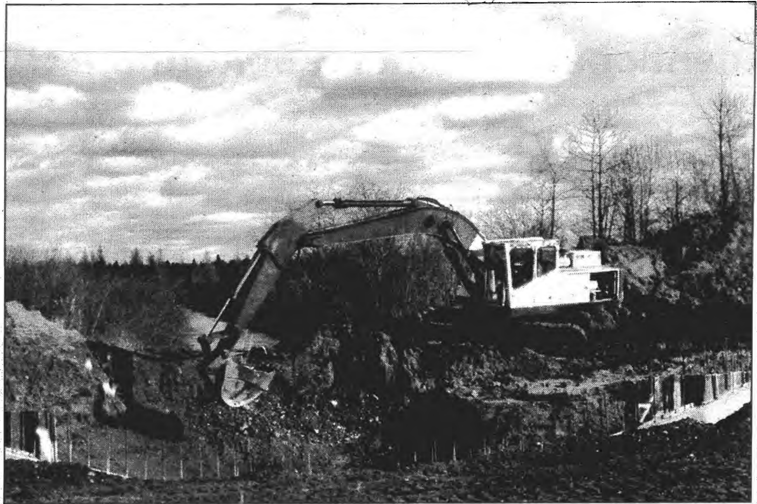
Building a berm next to the water control structure at Deadfish lake. Water flowing from the lake to the ditch (background) is diverted around the construction site. (Photo by C.O. Rasmussen)
