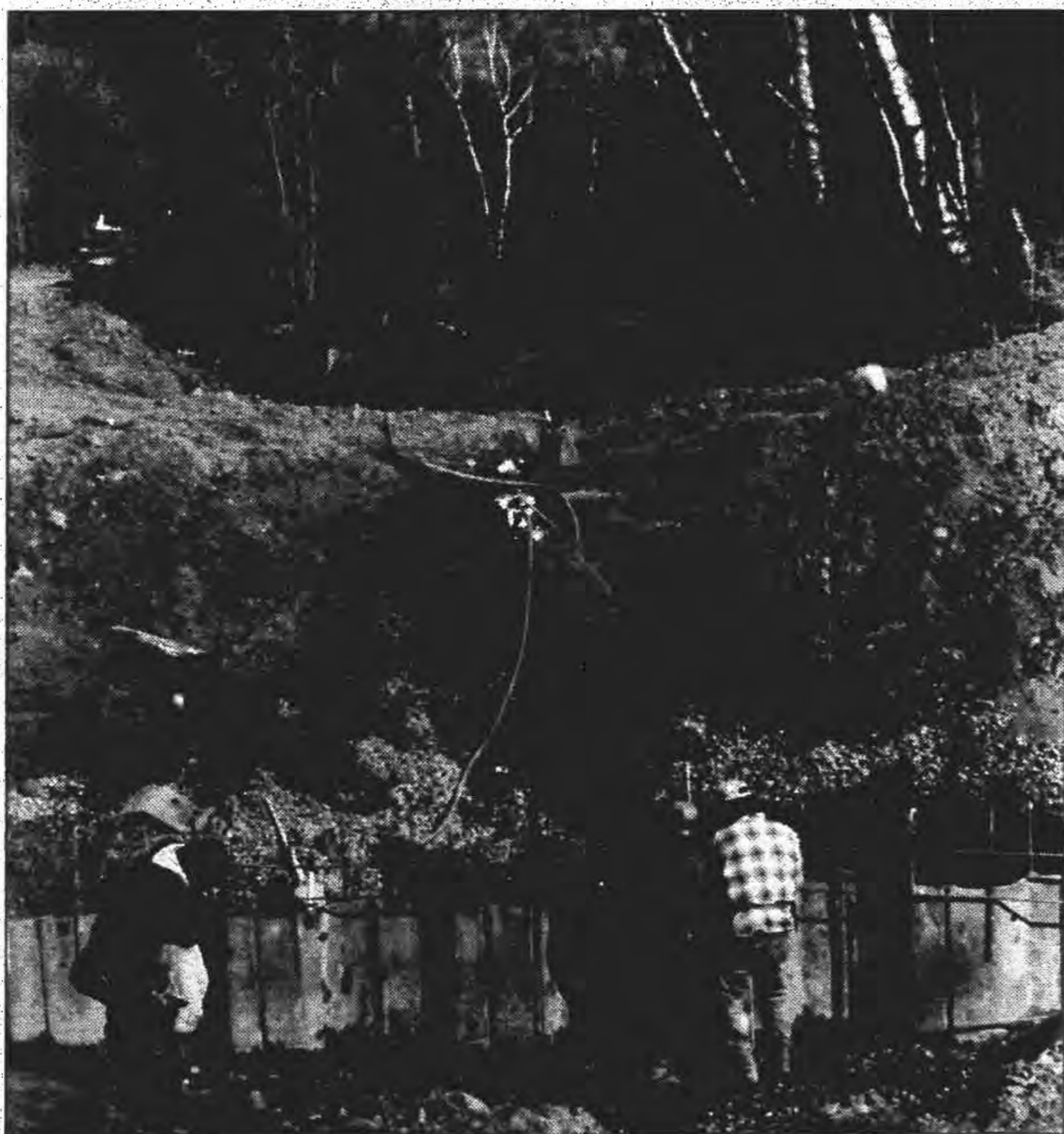
Construction workers install sheet piling at the Rice Portage lake outlet. The piling will reinforce the water control structure and help prevent seepage. (Photo by C.O. Rasmussen)
