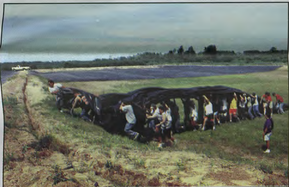
With help from the local youth group, Bad River hatchery technicians install a liner on a walleye rearing pond.
