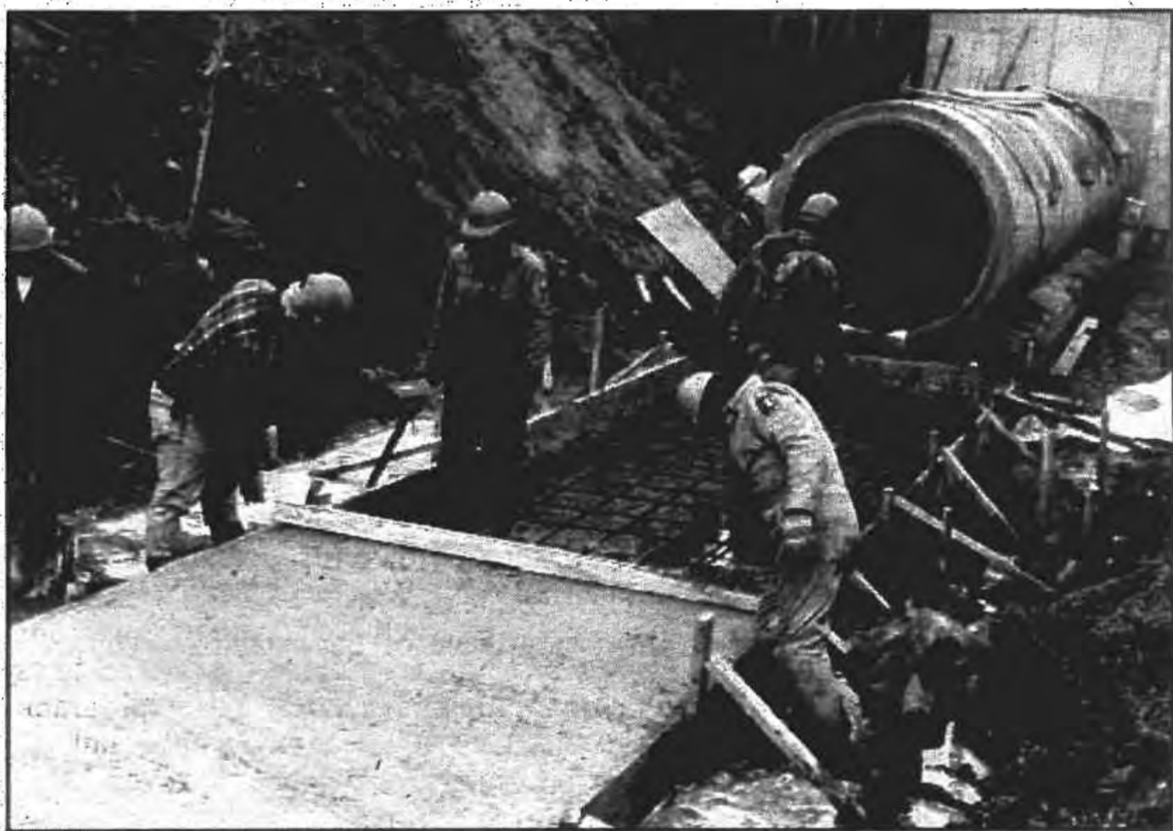
US Forest Service construction workers pour the concrete footing for the new water control structure at Wilson Flowage. (US Forest Service photo)
