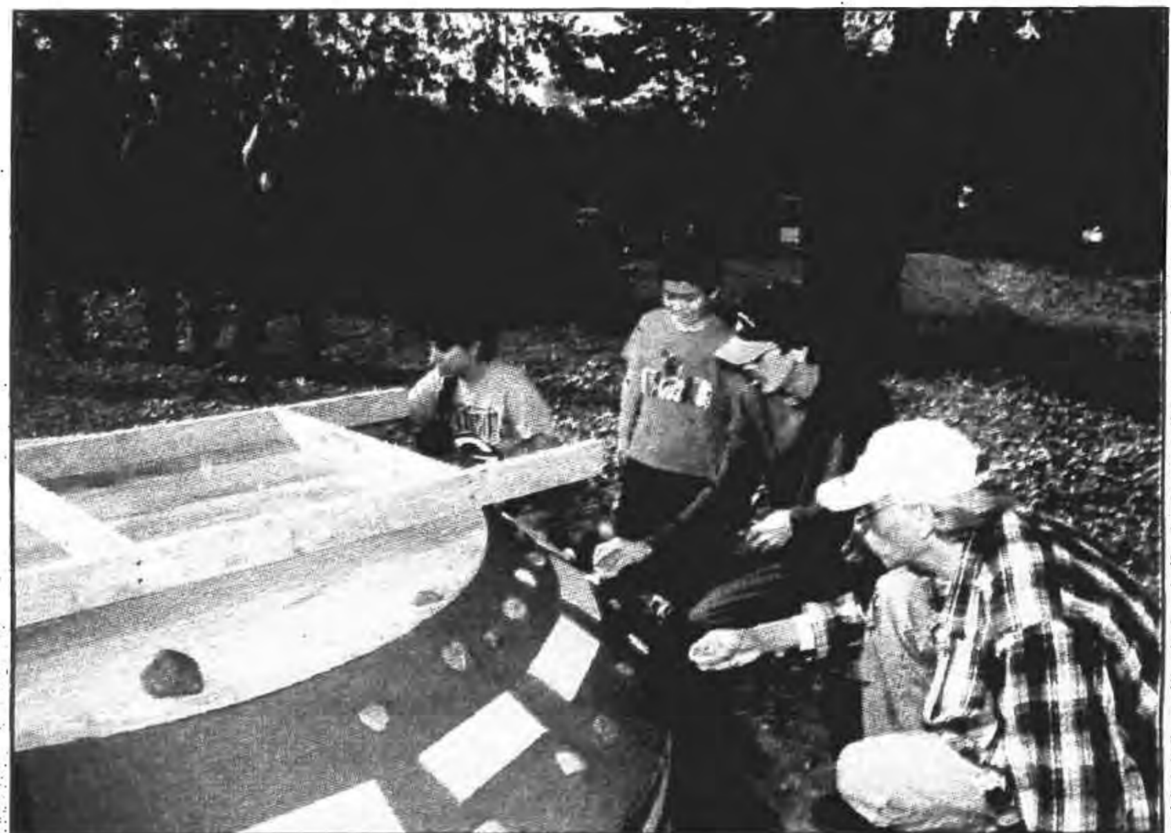
Placing grandfathers (stones) from ten Chippewa reservations into the base pedestal of the Sandy Lake Tragedy Memorial monument required many hands. Quickly drying concrete made fast work a necessity. Helping with the project are Fred Ackley, Mole Lake; Eugene Van Zile and son Roland, Mole Lake, and Gigi Cloud, GLIFWC. (Photo by Sue Erickson)
