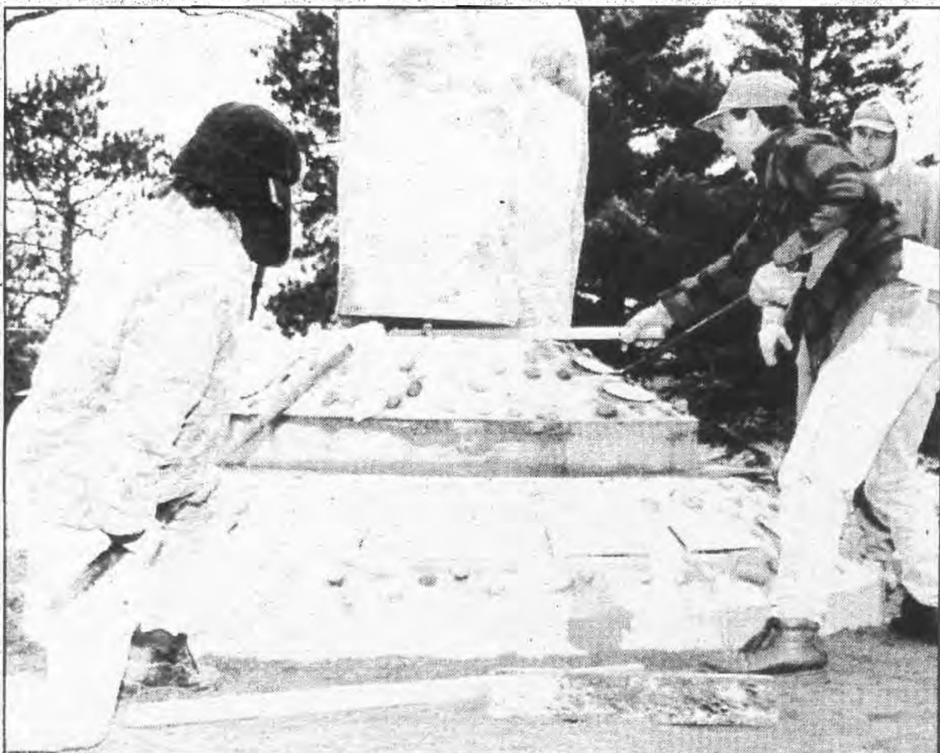
Bruce Goman, Mille Lacs Development Inc., and Jim Zorn, GLIFWC policy analyst, lower the boulder onto the pedestal of the Mikwendaagoziwag Monument last fall. Earlier in October the two-tiered pedestal was poured and the Grandfathers from 11 Ojibwe bands set into the concrete. (Photo by Charlie Otto Rasmussen)
