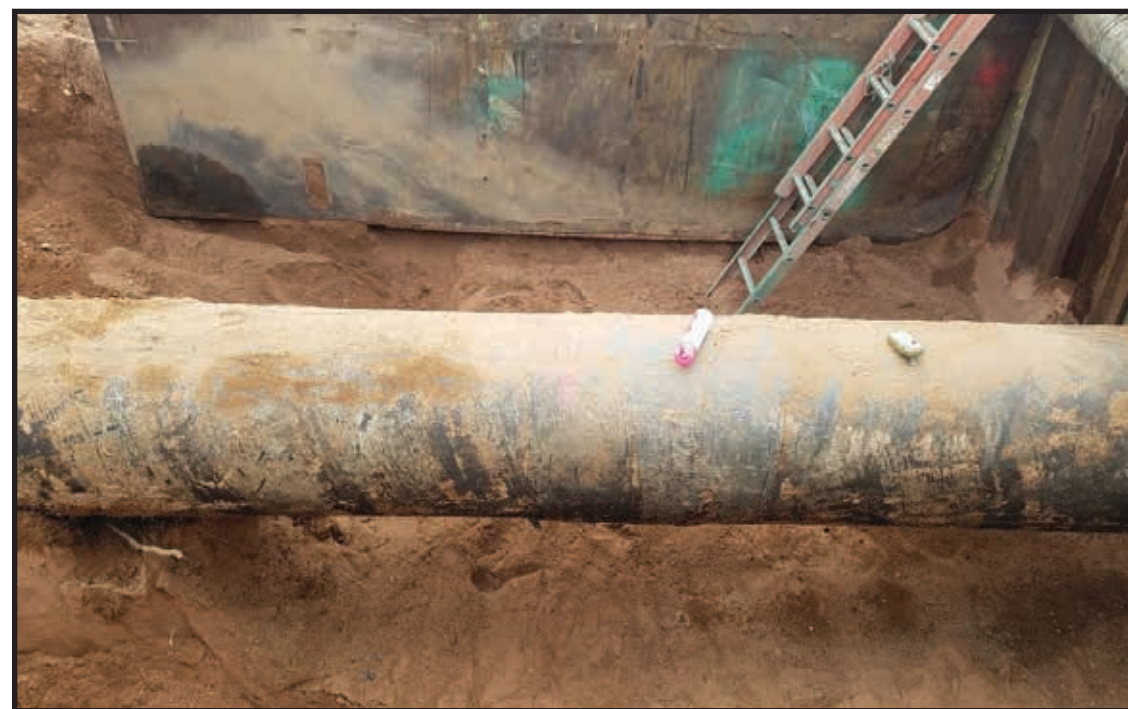
Line 5 pipeline exposed during an integrity dig in the Chequamegon-Nicolet National forest. Note the sandy soils in the excavated area. (D. White photo)
