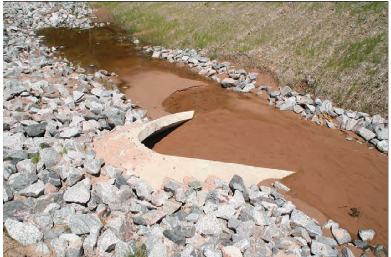
Undersized sedimentation basin along a mine haul road. The sediment will need to be removed for the basin to work as intended.
