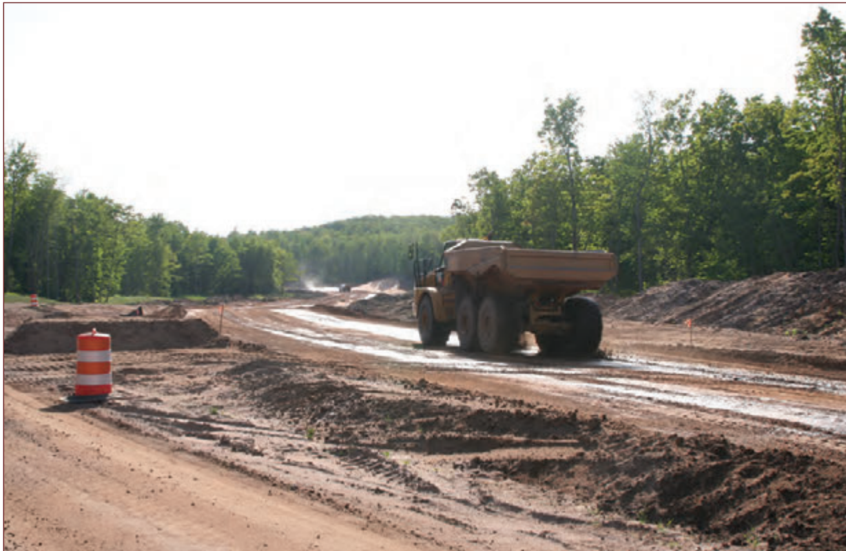
A mining haul road constructed after the Eagle mine was permitted in Michigan.
