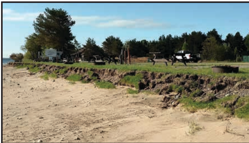
Coastal erosion at Bay Mills Indian Community near a campsite on the reservation. (Photo by Sara Smith, College of Menominee Nation Sustainable Development Institute.)
